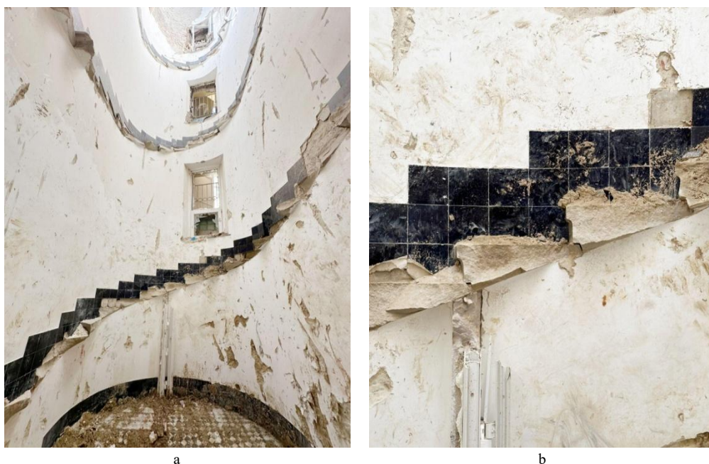
Fig. 7. The main stone staircase at 44 Konovaltsia Street, ruined by the attack: general view (a) and close-up (b). Documented on 04 September, 2024 (photo: Mariana Kaplinska)
