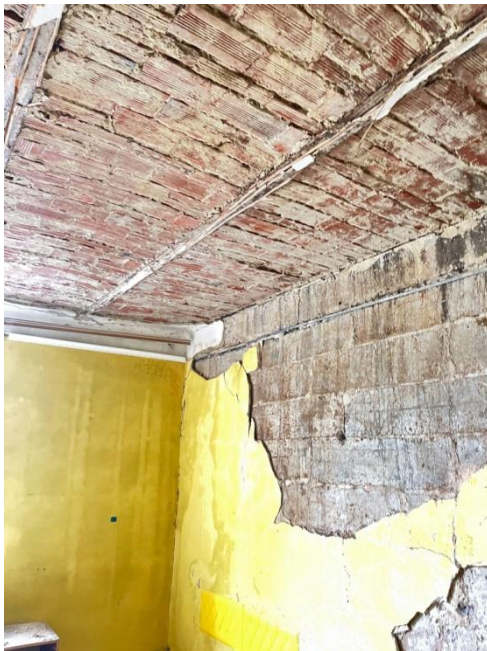
Fig. 15. Hollow brick jack arch floor structure on metal I-beams and a gypsum block partition in Building No. 64 on Stryiska Street after the missile strike, documented on 20 October 2023. (photo: Ihor Bokalo)
