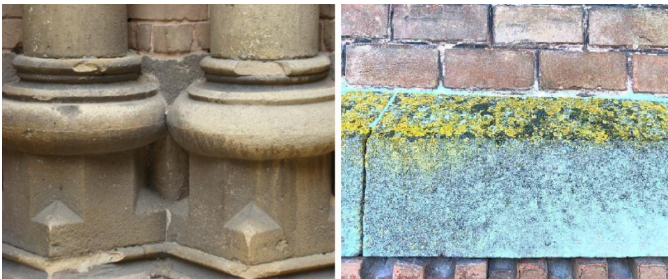
Fig. 4. Chemical and biological damage to the limestone surface on the Seminary Complex's facades (photo by I. Korotun, 2026)
