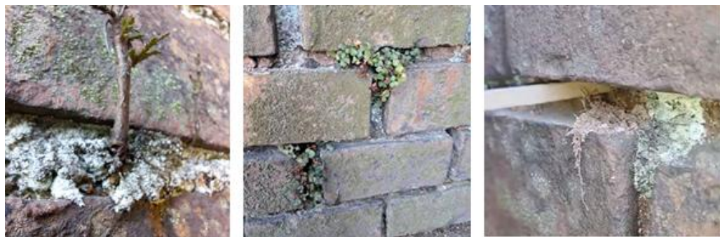
Fig. 2. Destruction of seams and brickwork surfaces by plants and the process of their removal (photo by K. Varvanych, 2025)
