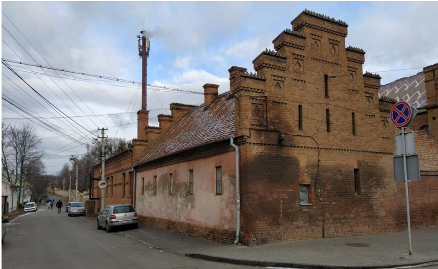
Fig. 1. Wetting and contamination of the facade surfaces of the outbuildings of the Seminary Building due to capillary wetting
