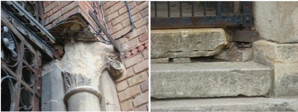
Fig. 5. Destruction (stone body's rupture) of limestone from contact with the gate iron fasteners. Gallery of the Seminary Building of the Residence of the Metropolitans of Bukovina and Dalmatia (photo by I. Korotun, 2015)
