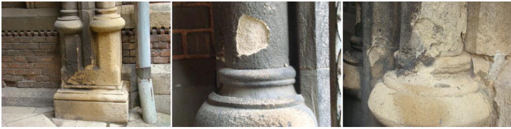
Fig. 6. Structural changes and destruction of limestone surfaces: "wild patina." Gallery of the Seminary Building of the Residence of the Metropolitans of Bukovina and Dalmatia (photo by I. Korotun, 2025)
