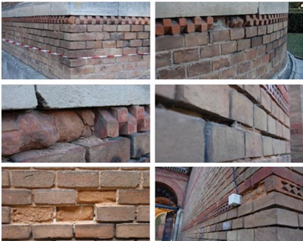
Fig. 3. Seams' weathering and decorative and masonry elements' destruction under the atmospheric factors' influence. Seminary building of the Bukovina and Dalmatia Metropolitans' Residence. Research of the Yuriy Fedkovych Chernivtsi National University Master students (Yerokhin B., Ilichuk M., Mazur O., supervisor I.V. Korotun, 2015)
