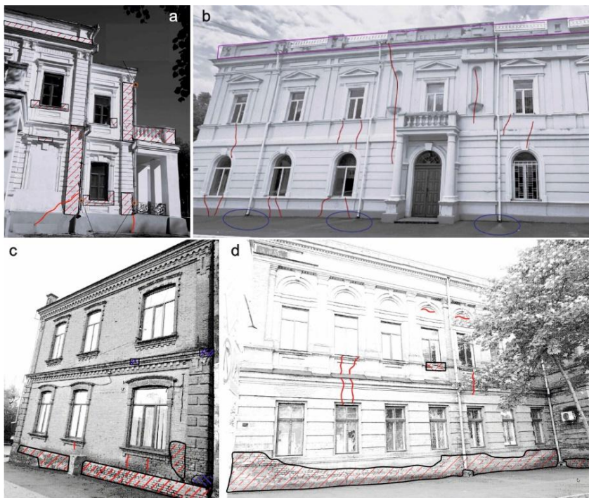
Fig. 3. Excerpts from inspection reports of damaged buildings, where red lines show cracks and red hatching shows masonry destruction: a – Andrushivka Lyceum No. 1 with a primary school (Zhytomyr region); b) Balta Oles Gonchar Lyceum No. 1 (Odesa region); c) Izmail Lyceum No. 1 (Odesa region); d) Izmail Gymnasium No. 2 (Odesa region)
