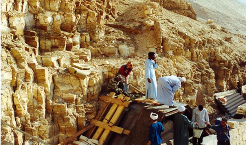
Fig. 2. The Sun Cult Complex. Shrine of Anubis and the northern wall of the courtyard during the project. State during conservation work in 2005.
