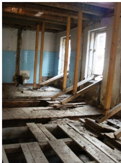
Fig. 12. Interior of the first floor—preserved construction of the outer walls—Hotel Zagreb building, CPNMBiH (2011)
