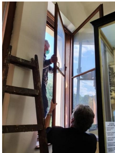
Fig. 8. Field research on the authentic window from the Austro–Hungarian period on the south facade of the Pavilion of Natural Sciences, phase II, CPNMBiH. Photo by Mak Bećirbašić, 2020
