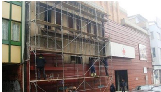
Fig. 4. Bosnian Red Cross Society building: Transferring the sheet from the facade onto the roof, CPNMBiH (2015)
