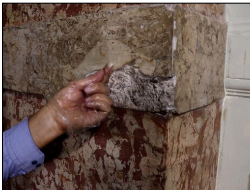
Fig. 4. deterioration phenomena forms in Scagliola at Zafaran palace
