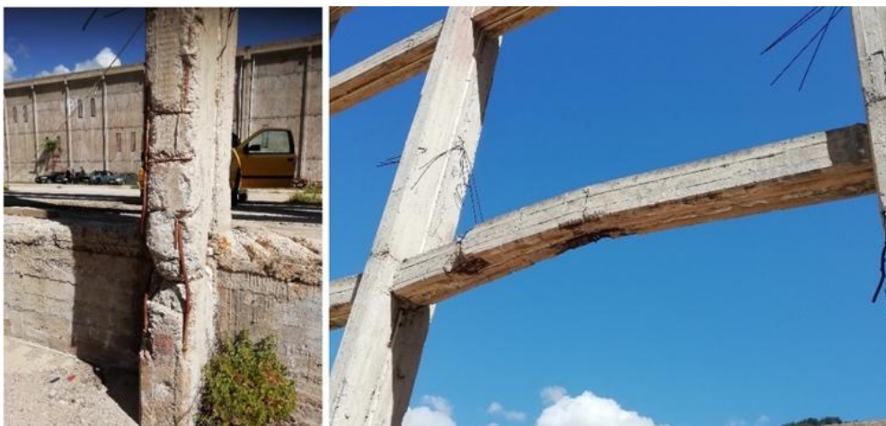
Fig. 27. Localized concrete failure, corrosion and failure of shear reinforcement, and buckling of longitudinal reinforcement
