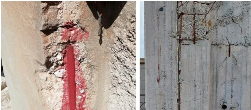
Fig. 25. Spalling and corrosion damage on the building's columns and walls
