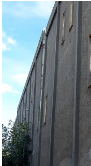
Fig. 8. Photograph of the leaning wall
