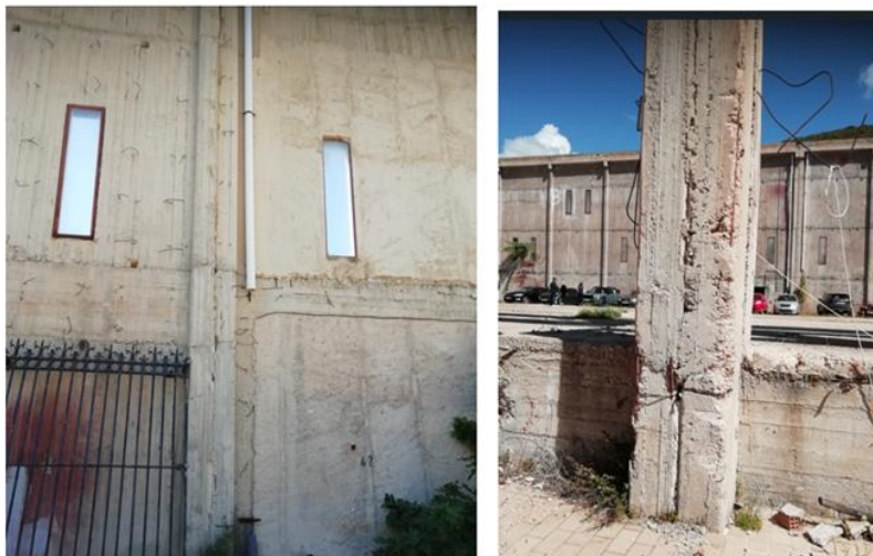
Fig. 26. Deterioration of the concrete cover and exposure of steel reinforcement at the joints
