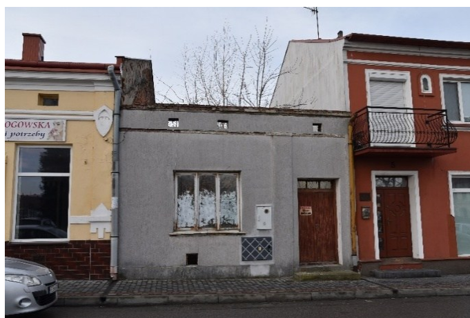
Fig. 14. View of a section of the western frontage of the market square and the façade of the neglected and degraded Rynek 4 building, where renovation works have been started and interrupted. Existing condition
