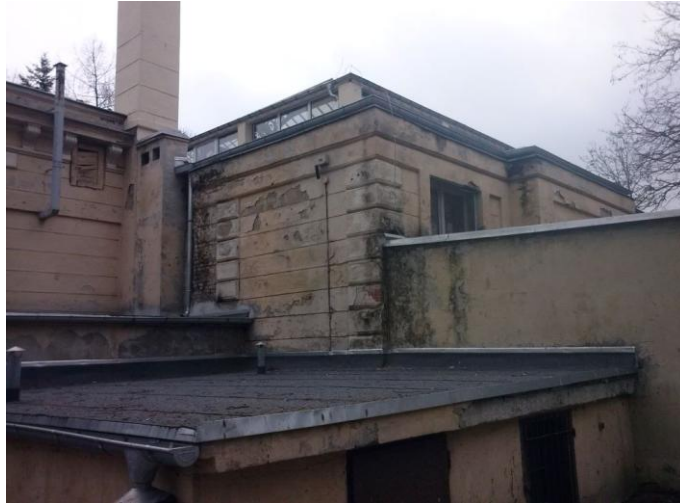
Fig. 6. Wrocław Zoo—Bird House—external view, state before renovation (photo by Beata Pawelec, Creoprojekt)
