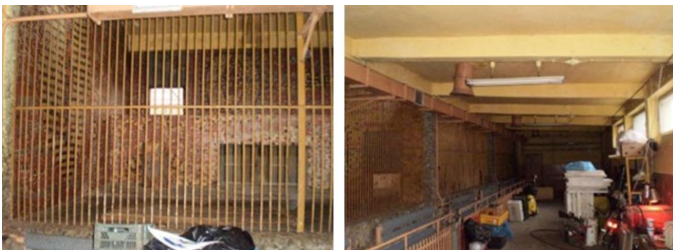
Fig. 21. Cracow Zoo - Existing condition of the interiors of the big cat pavilion before its demolition in 2009 (photo by K. Wawer/P. Redmerski)
