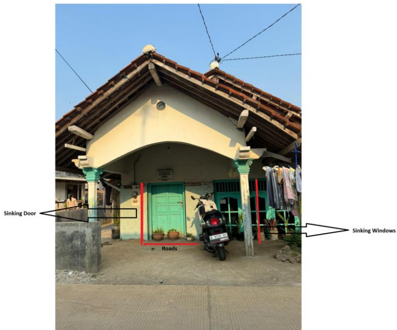
Fig. 8. Field documentation shows an example of sinking houses, where it can be seen in this image that only part of the house door is visible, as the rest has sunk into the ground.
