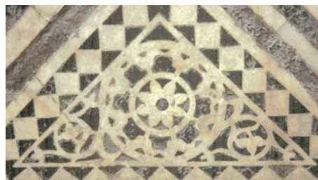
Fig. 16. One of the tiles from the baptistery flooring, featuring phytomorphic geometric decoration ( southeast sector )
