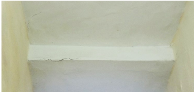
Fig. 12. Damage to the floor beam due to the impact of the blast wave, Zolochiv school No. 1, Lviv Region
