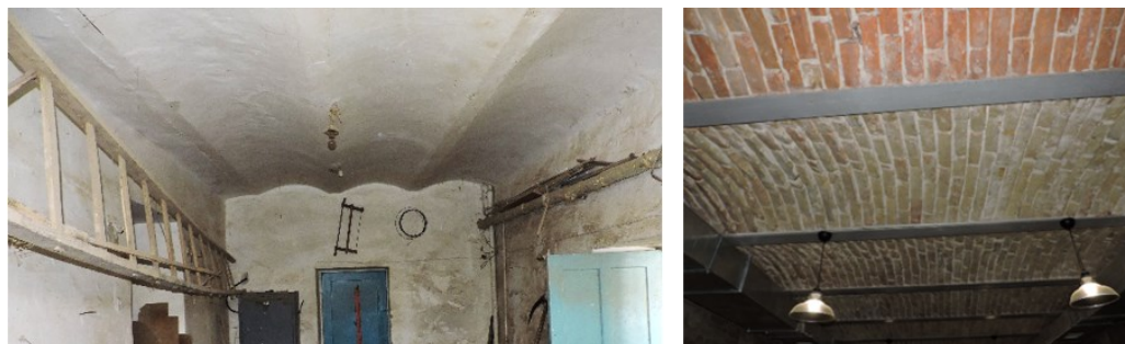
Fig. 14. Metal beams in the ceiling in basements (Zolochiv school No. 1, Lviv Region)
