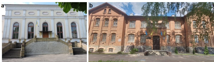
Fig. 2. Examples of historical buildings that were damaged as a result of military actions, in particular from explosive (dynamic) impacts either from rockets or UAVs: a – Zolochiv school No. 1, Lviv Region 1; b – Onufriiv Lyceum (building No. 1), Kirovohrad Region
