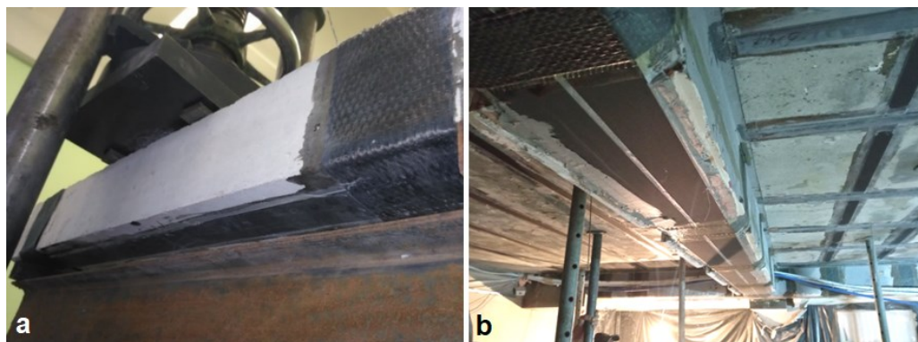
Fig. 13. Span structures reinforced with high-strength carbon materials (FRP) : a - reinforced concrete beam in the process of experimental research (mounted on a press before testing); b – reinforcement of the beam slab of the floor at the construction site
