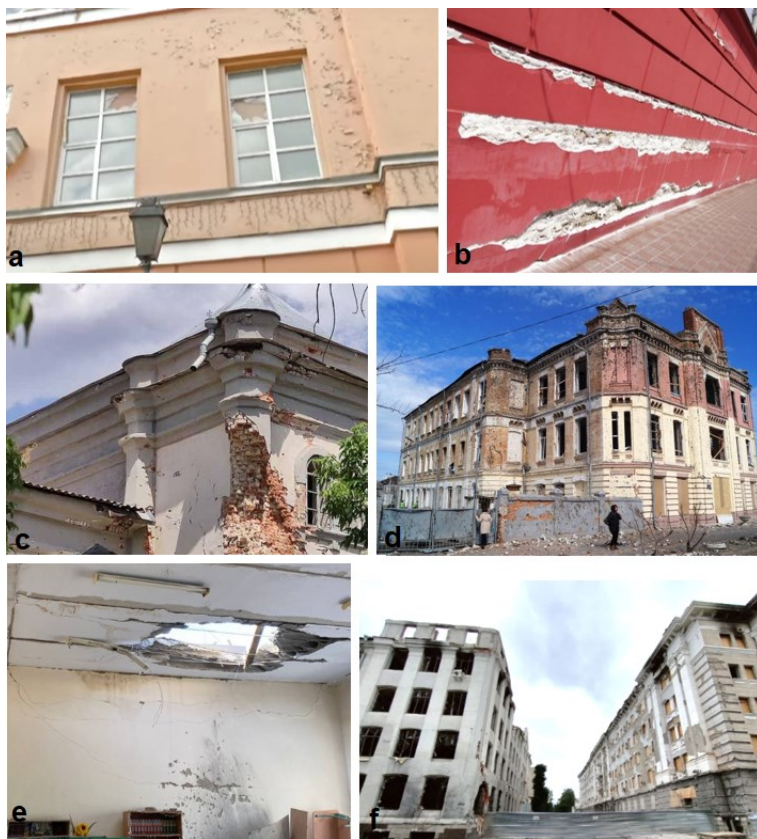
Fig. 3. Damage to structures of historical buildings of educational institutions: a, b, d, f – damage to facades; c, d, f – damage to masonry walls; e, f – damage to floor slabs; f - damage to the roof structures; namely: a-b – The main building of the Taras Shevchenko National University of Kyiv; c - Borivske Church of St. Nikolas, Luhansk region; d - Kharkiv School No. 7; e - Vysokopil Lyceum, Kharkiv Region; f - V. N. Karazin Kharkiv National University [https://www.5.ua/kyiv/raketnyi-udar-po-kyievu-naskilky-sylno-postrazhdav-universytet-imeni-tarasa-shevchenka-290134.html; https://culturecrimes.mkp.gov]
