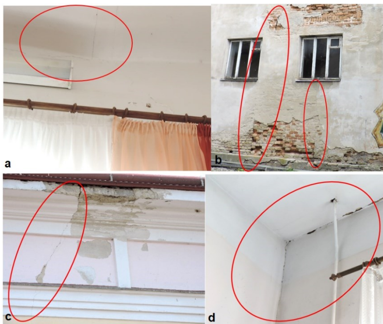
Fig. 5. Occurrence of cracks after dynamic explosion impacts: a – in the joints of floor slabs; b, c – in the walls; d - in the joints of the walls and ceiling, where: a - Onufriiv Lyceum (building No. 1), Kirovohrad region 1; b, c, d – Zolochiv school No. 1, Lviv Region
