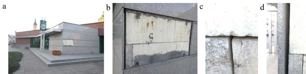
Fig. 2. The bank in Byczyna: a – general view; b-d – the quality of the wall facing
