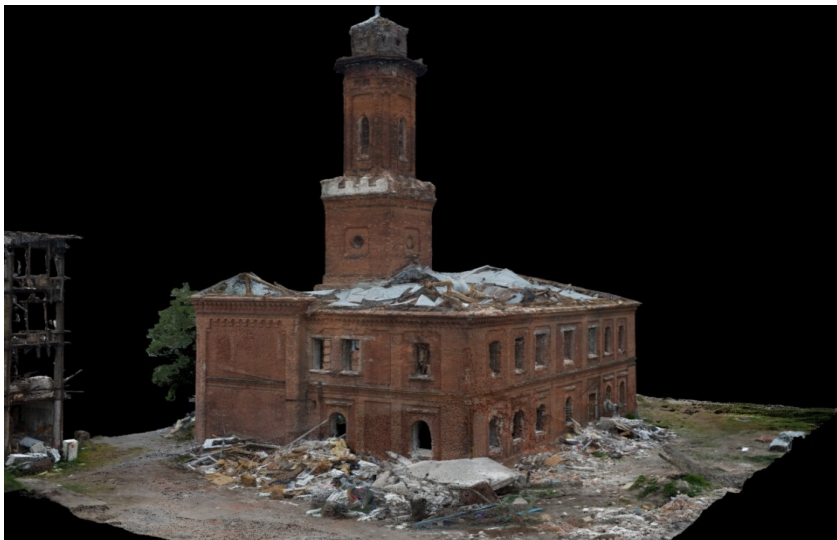
Fig. 1. A three-dimensional digital model of the fire station in Zaikivka at 25 Kvitkivska Street, Kharkiv (1886), created by Serhii Revenko as part of the SCAN UA project ( https://scanua.com/firedepartment/ )
