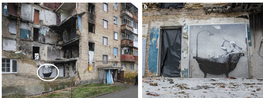
Fig. 4. Mural Banksy in Gorenka. Photo by G. Garanich (Reuters), H. Shpakova: a - November 2022; b - after installing the protective screen, February 2023
