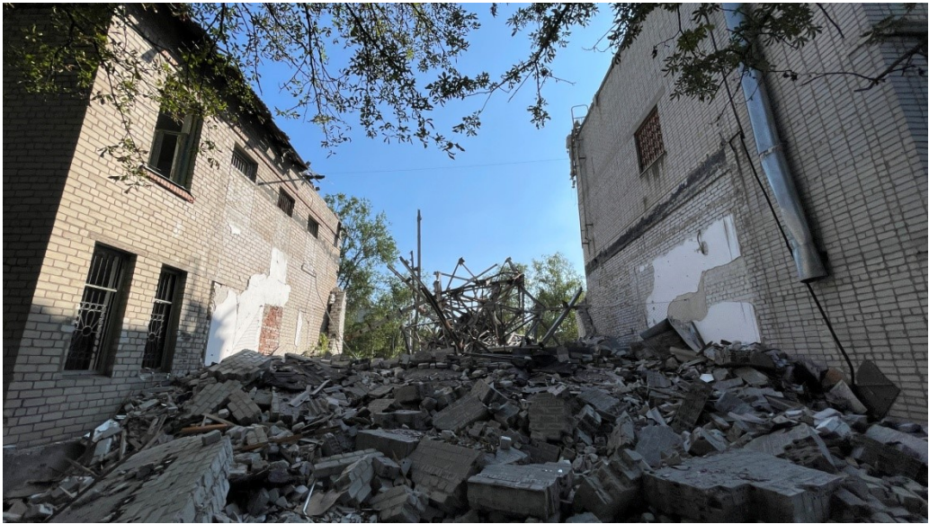
Fig. 11. Demolished building in Kramatorsk [Photo by Serhii Belinskyi, 2023]
