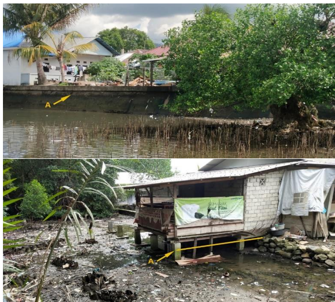
Fig. 6. Residential area with seawall as coastal defense structure at the back of the mangrove area at Passo (above) and Waiheru area (below). The tip of arrow A points to the sea level position at the high tide. Photo: March 2022
