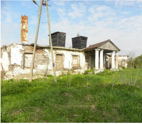
Fig. 17. The disastrous condition of the manor house in Jaszczów in 2011
