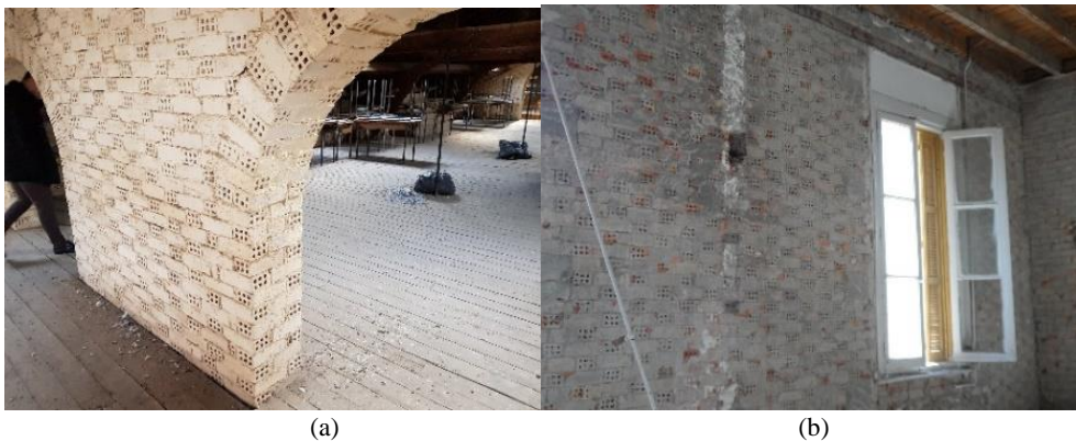
Fig. 9. Perforated, baked earth bricks: a) Secondary load-bearing wall; b) Main load-bearing wall
