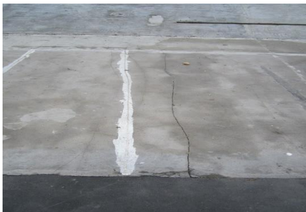
Fig. 7. Cracks on the bicycle track
