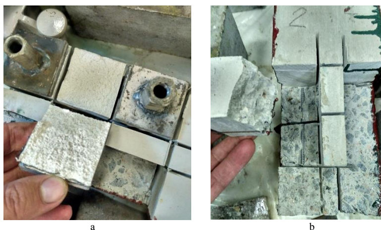
Fig. 12. Cohesive destruction: a – material in Mapecoat TNS Base Coat layers; b – concrete material of the bridge
