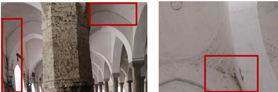
Fig. 11. Visible joint cracks of Shat Gombuj Mosque
