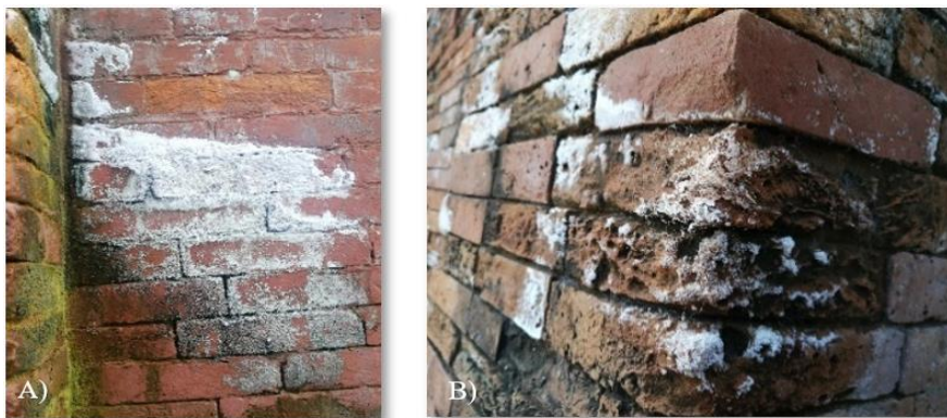
Fig. 8. Crystal formation of salt and erosion of the building materials in Khalifatabad
