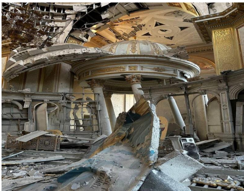
Fig. 1. Destruction of the main cathedral of the Eparchy of Odesa founded in 1795.
