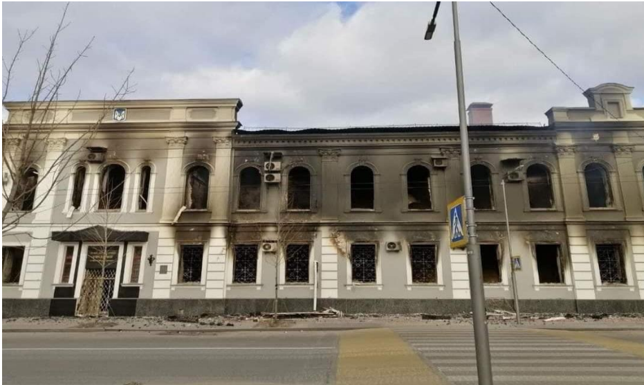
Fig. 3. Damage to a historical monument, the former Chernihiv District Court building, built in 1904.
