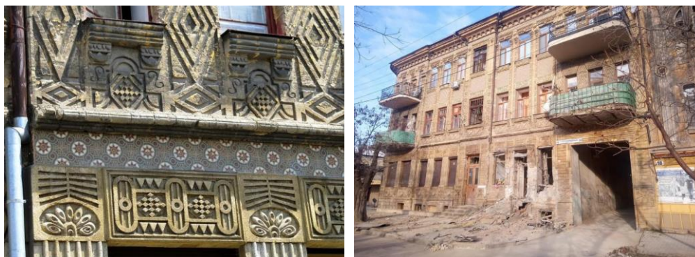
Fig. 2. Damage to the house of Peruvian merchants in Kherson after Russian shelling, built in 1905 in Kherson
