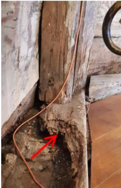
Fig. 22. Degraded sill plate in the chancel
