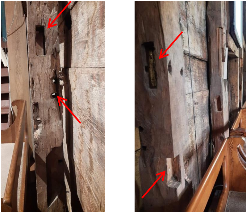
Fig. 20. Notches and dowel holes weakening the columns in the north wall of the nave
