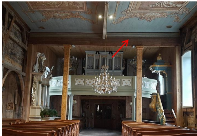
Fig. 4. View of the three-span beam supporting the nave girder from the choir section
