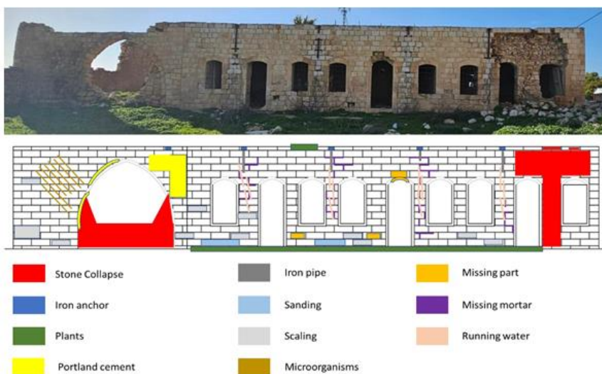
Fig. 13. Shows the condition assessment of Al-Rawabdeh building and the extent of deterioration of the front facade
