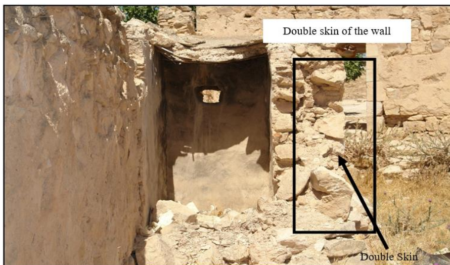
Fig. 8. Schematic illustration of wall component with two outer layers and gravels filler in between
