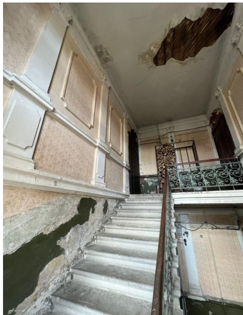
Fig. 6. The dilapidated condition of the entrance space of a residential building located at 28 Hetmana I. Mazepy Street, Ivano-Frankivsk.
