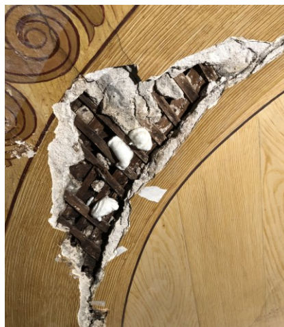
Fig. 5. Damage from growing salt crystals due to overwetting
