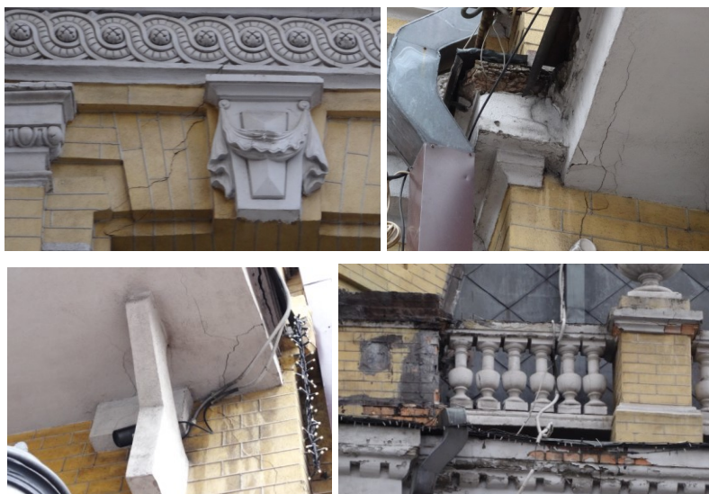
Fig. 6. Typical facade damages. Photos by Oleksandr Molodid, 2021
