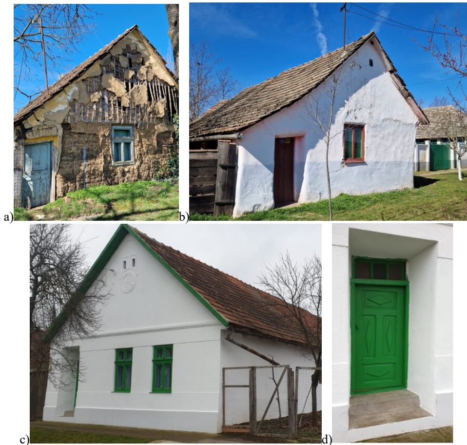
Fig. 9. Examples of Romanian rural heritage - Mailat village, Vinga commune, Arad County: a) Traditional house in an advanced state of decay, suitable for consolidation and repair works using traditional materials and techniques; b) Traditional house (in use); c) and d) Traditional house renovated with appropriate materials to preserve the architectural specificity
