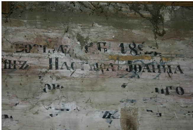
Fig. 16. The foundation inscription on the southern wall of the women's porch, photo T. Tomaszek
