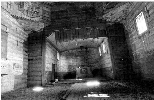
Fig. 28. Interior of the church in Mięksisz Stary (from the side of the nave towards the sanctuary) after the dismantling of the iconostasis—see the traces showing where the iconostasis was supported by the wall, 1987, source: the archives of the Department of Eastern Church Art in the Museum of the Łańcut Castle
