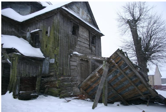
Fig. 11. Collapsed porch adjacent to the women's porch from the west, photo T. Tomaszek
