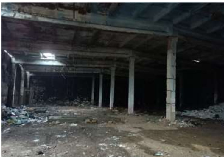
Fig. 2. The damaged workshop of the enterprise in Bakhmut (Donetsk region).
