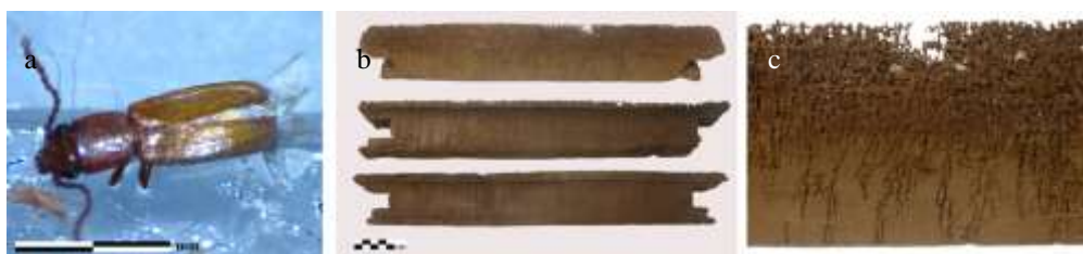
Fig. 4. Powder post beetle ( Lyctus brunneus ): (a) Adult powder post beetle (b) Remains of a wooden coffin attacked by powder post beetles (c) Corridors, exit holes, and heavy damage caused by powder post beetles
