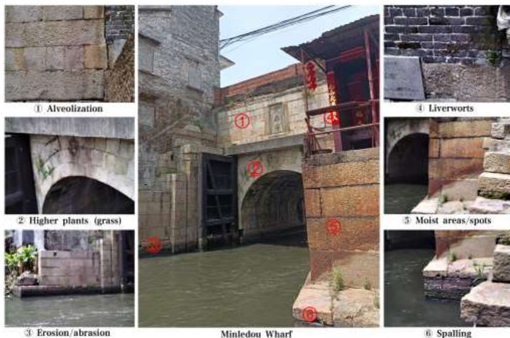
Fig. 1. Six types of damage and weathering in Minledou Wharf
