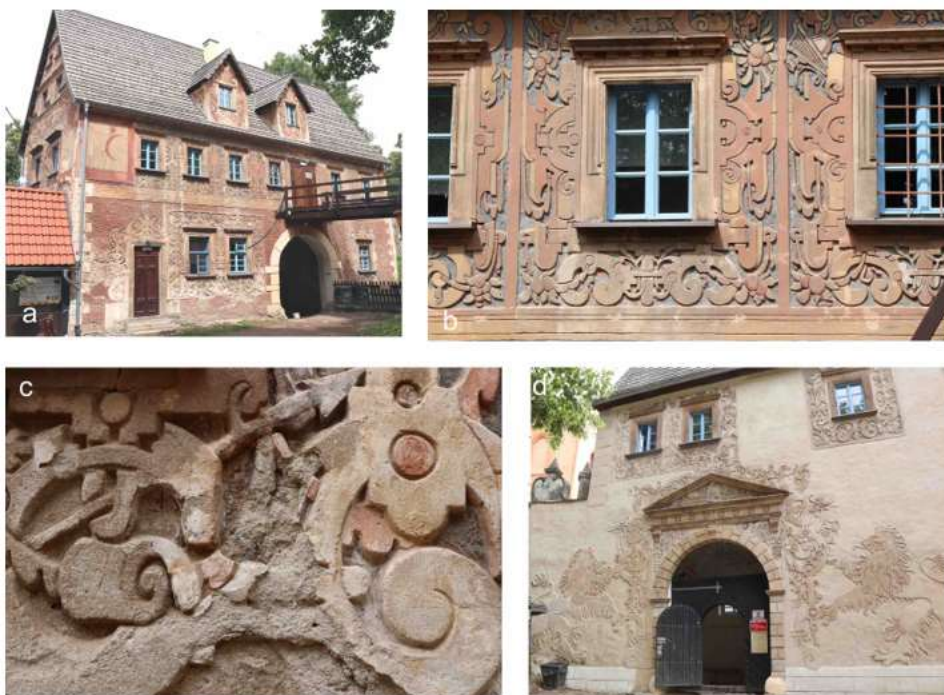
Fig. 14. Grodno Castle in Zagórze Śląskie, sgraffito decoration of the gatehouse from the 4th quarter of the 16th century: (a) view from the outer ward, (b) window frames on the 1st floor from the side of the outer ward after two restoration works in 1903-1906 and 1957-1959, which received vivid colors that were similar to the original ones, (c) state of preservation of the sgraffito decoration on the ground floor, (d) sgraffito-stone gate portal, as seen from the outside (from 2015), which was stripped of color after subsequent restoration works, photo by Agnieszka Gryglewska (used with permission)
