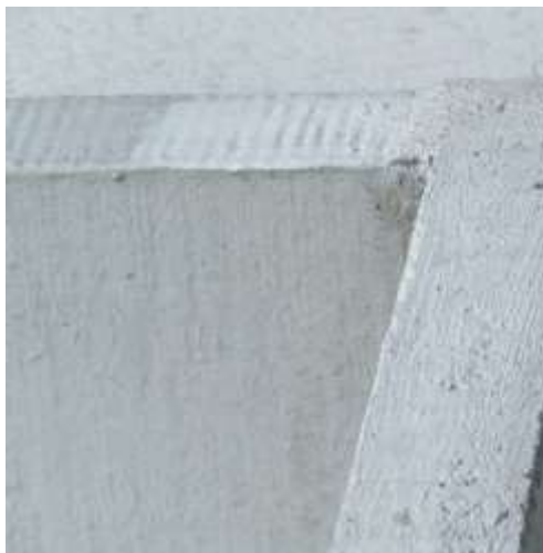
Fig. 17. Infill housing development - a residential building right corner, dating back to 1961 at 28 Czerwca 1956 nr 138. A study of stone damage due to the use of improper facade paint. No possibility of air reaching the structure of the material. Materials prepared by the authors
