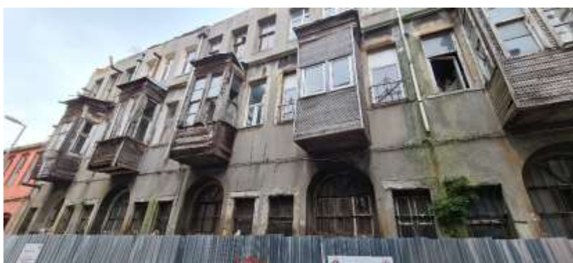
Fig. 5. Fatih-Kumkapı area: deteriorated masonry row houses (listed civil architectural examples)
