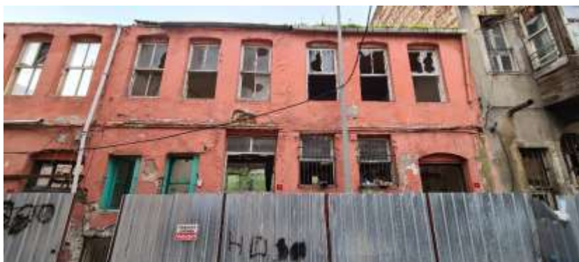
Fig. 4. Fatih-Kumkapı area: deteriorated masonry row houses (listed civil architectural examples)
