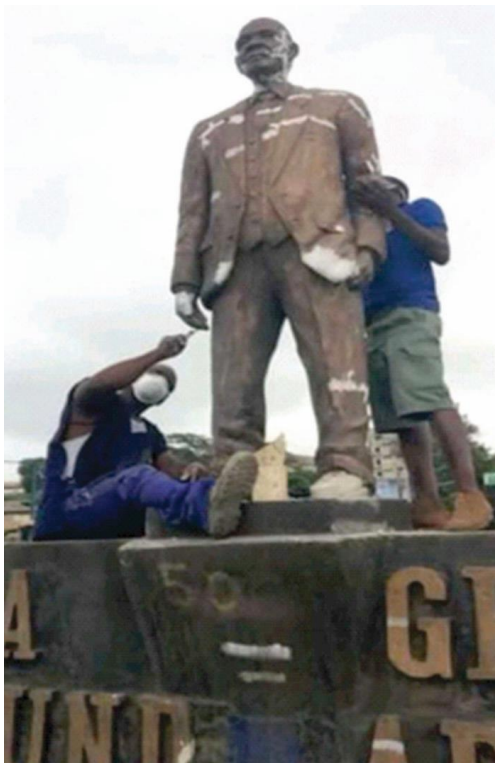
Fig. 7. Practitioners restoring the sculpture of Paa Grant with cement mixture (penetrating sealants) and enamel paint
