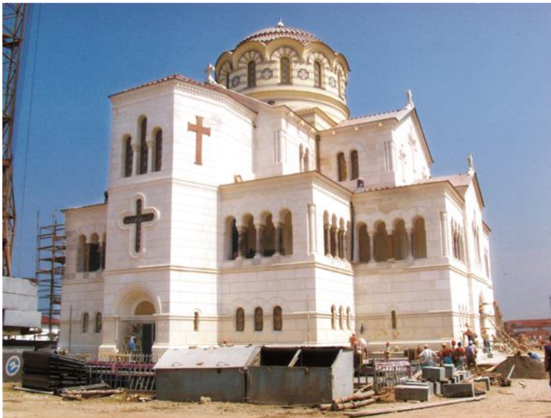
Fig. 4. The state of the cathedral after the completion of the first stage of restoration (July 25, 2001). Photo from the stocks of the Ukrrestavrtsiia Corporation
