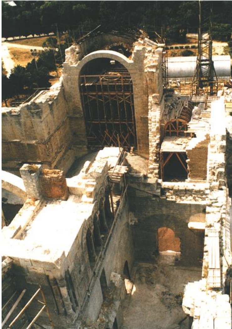
Fig. 2. The beginning of the cathedral walls restoration. Photo from the stocks of the Ukrrestavratsiia Corporation
