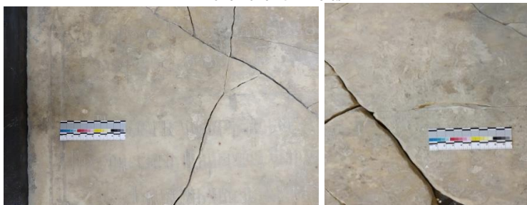
Holes are the weakest spots on the stone surface that fall off and separate from the stone
