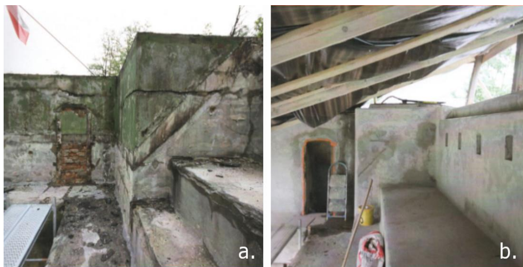
Fig. 5. The condition of the shooting gallery after the disassembly of the roof (a.) and during conservatory works (b.).
