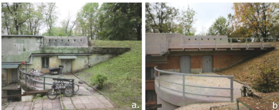
Fig. 6. Condition of the eastern elevation prior to the commencement of works (a.) and after their completion (b.). Visible repainting, cracks, and cavities in the brick wall, as well as altered brickwork and sizes of openings.
