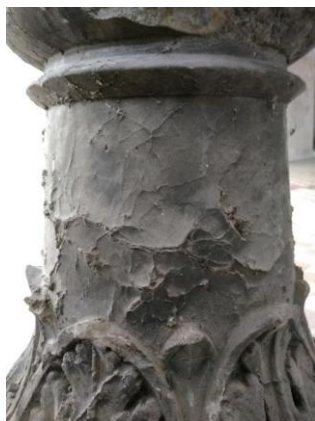
Fig. 10. Cleavage, cracks and dirt on the pedestal surface of the alabaster baptismal font
