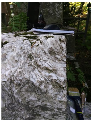
Fig. 2. Deep cracking of the stone
