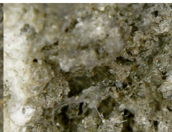
Fig. 14. Clusters of dirt. Surface formations confined to cracks
