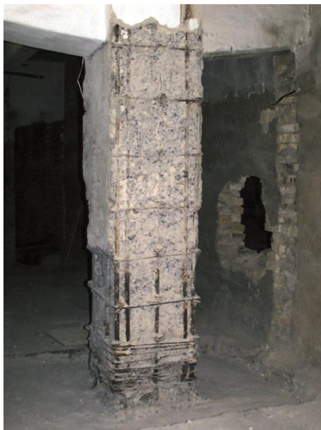
Fig. 1. Condition of the reinforced concrete column before renovation. Photo from the funds of the Ukrrestavratsiia corporation, 2001
