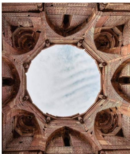
Fig. 2. Sky is visible from the inside of the Tomb of Iltutmish at Qutb Complex, Delhi, as the dome got broken off due to faulty architectural lapses. Photo credit: Anas Khan - unzip_delhi
