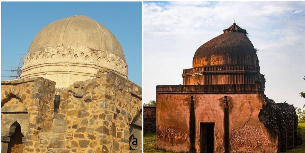
Fig. 3. (a) The Detail of cracks in the dome on the exterior surface of the tomb of Alia Darwaza, (b) The damaged dome of Salimgarh fort.
