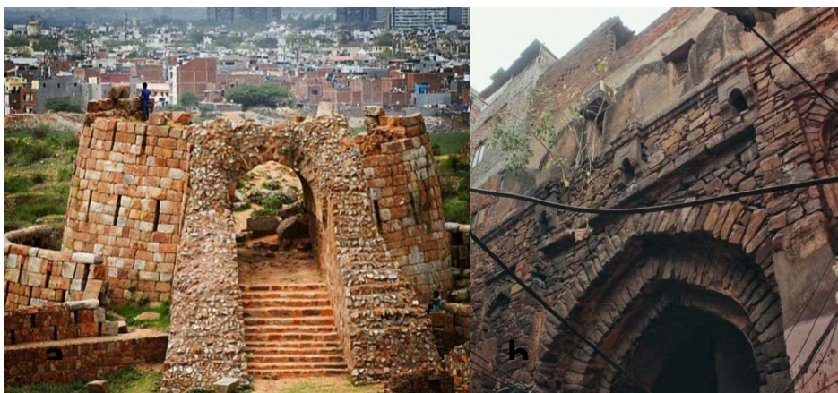
Fig. 5. Expanding encroachments within Tughlaqabad Fort, which is a ruined fort in Delhi built by Ghiyas-ud-din Tughlaq, the founder of Tughlaq dynasty. (b) Used and abused structure structure of Nabi Karim.
