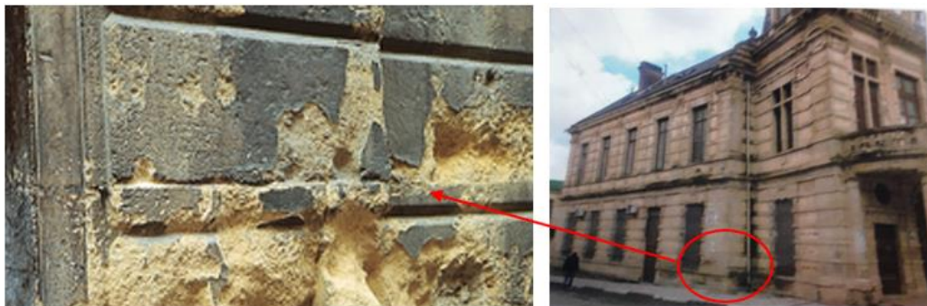
Fig. 4. Alveolization on the North Facade
