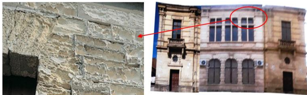
Fig. 5. Dissolution on the South East façade
